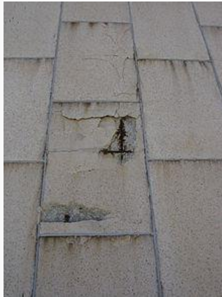
Detailed view of spalling.
